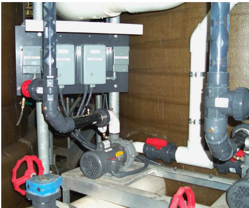
Fig. 3. Water pumped through a venturi injector (where ozone gas was suctioned into the flow) was then passed through an inline static mixer before being piped to the down flow bubble contactor.
