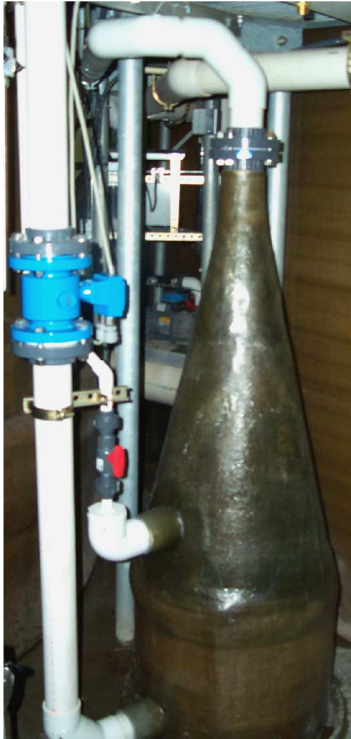
Fig. 4. A down flow bubble contactor was used to remove off-gas from the side-stream flow before it entered the UV irradiation chamber.
