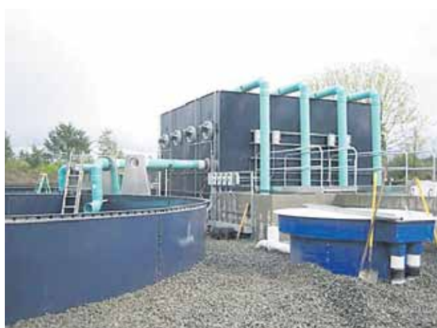
A new outside recirc system. The large tank in the back is the low-head biofilter.
